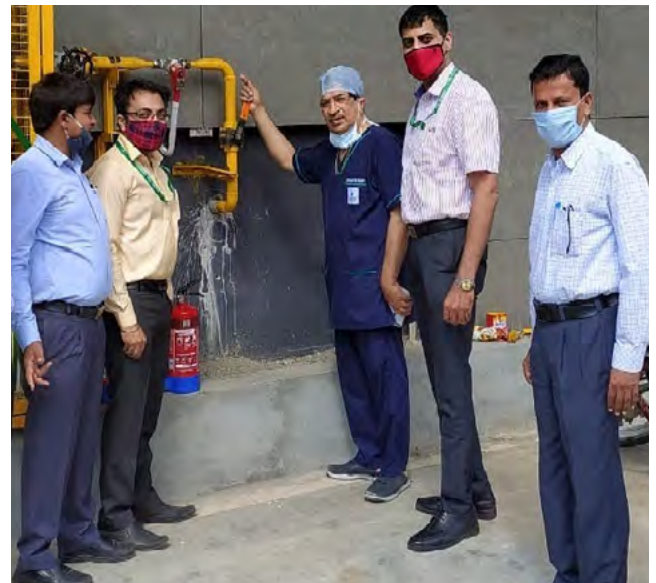
First Commercial PNG connection by Indraprastha Gas Limited in Muzaffarnagar, Uttar Pradesh, being commissioned at Vardhman Hospital, Muzaffarnagar.
