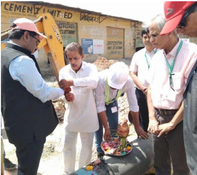
Shri Pawan Kumar, Director (Commercial), IGL inaugurating the project work on laying steel pipeline on NH-58 & 448 (Beawer to Kishangarh) in Ajmer, Rajasthan.
